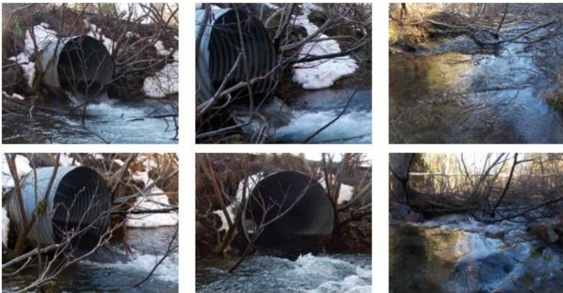
Figure 1: Photos of the 19 cm outflow drop before constructing the rock weir (top left and center) with their corresponding after photos following rock weir completion. (bottom left and
