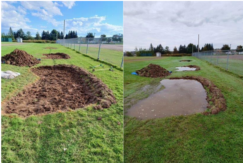
Figure 9: Hal Betts rain garden adjacent to the parking lot under construction. We are planning to finish this rain garden in the next spring/2024.
